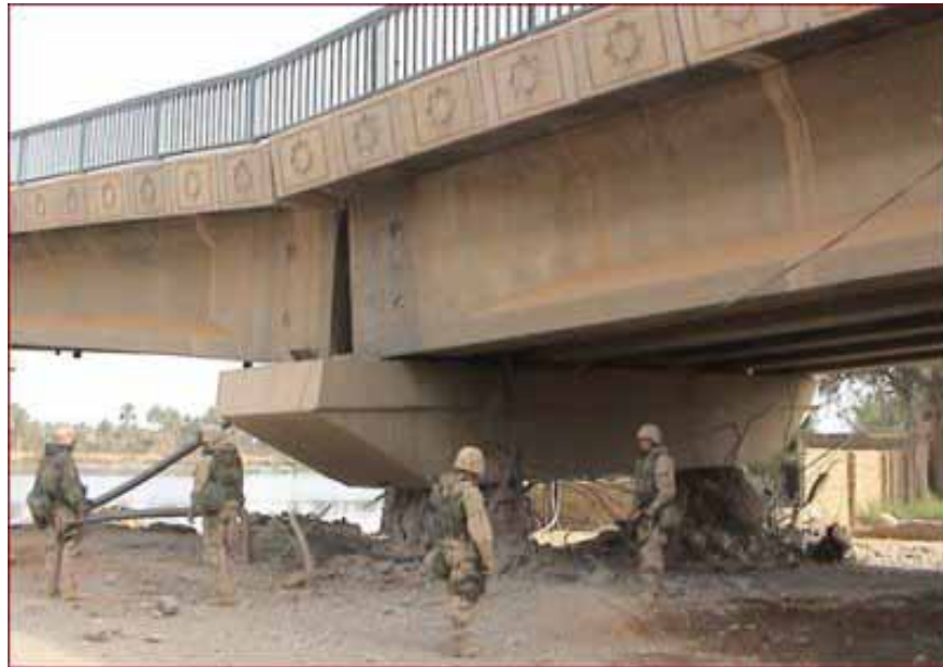
Figure 1.1 A bridge in Iraq damaged by a relatively small amount of explosives placed in a terrorist attack.
