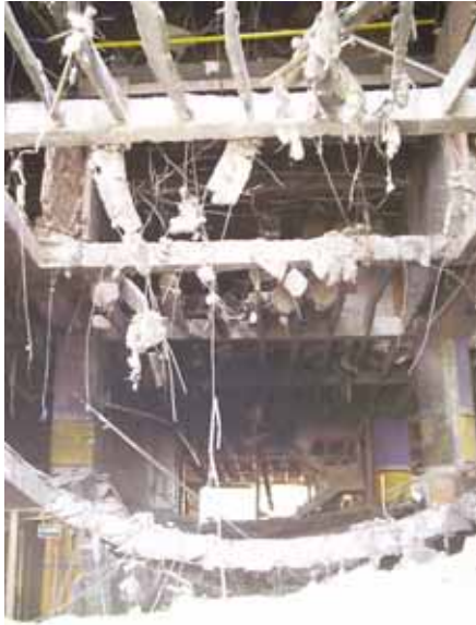
Figure 5.17: Damaged Club El Nogal Site. Undamaged column is pointed by an arrow.
