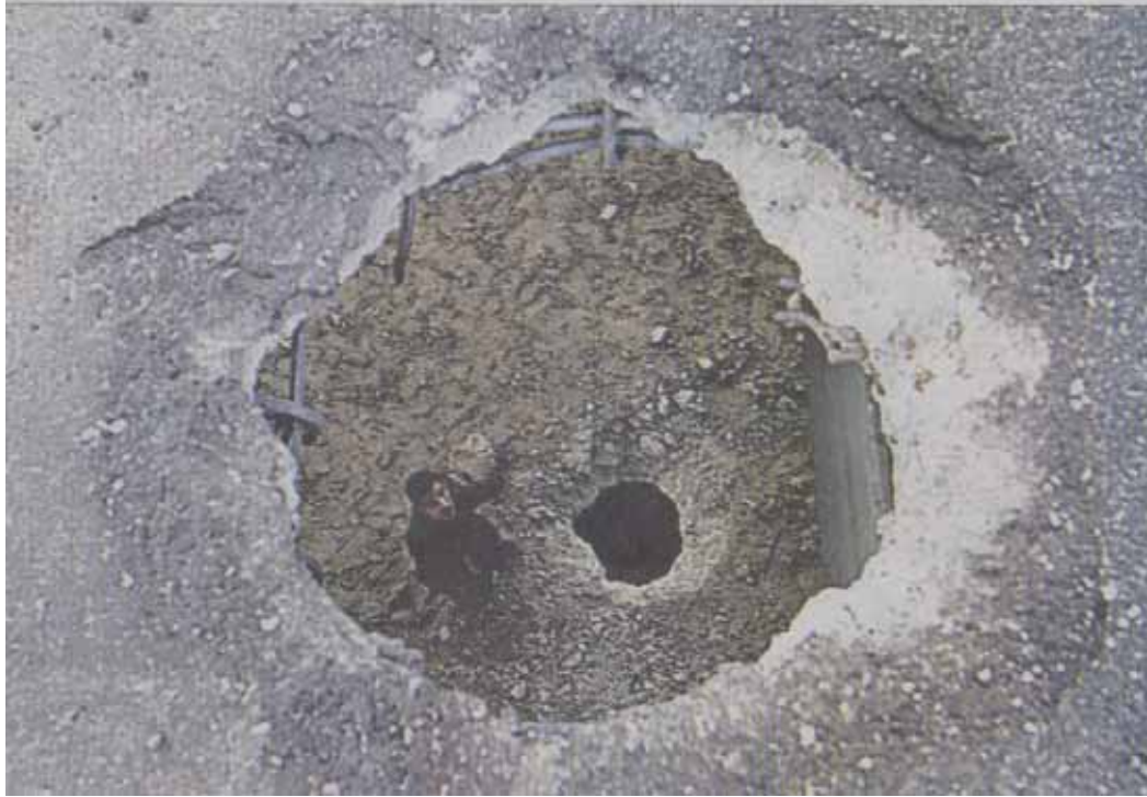
Figure 3.1. Damages to a Bridge in Palestine After a Missile Attack.
