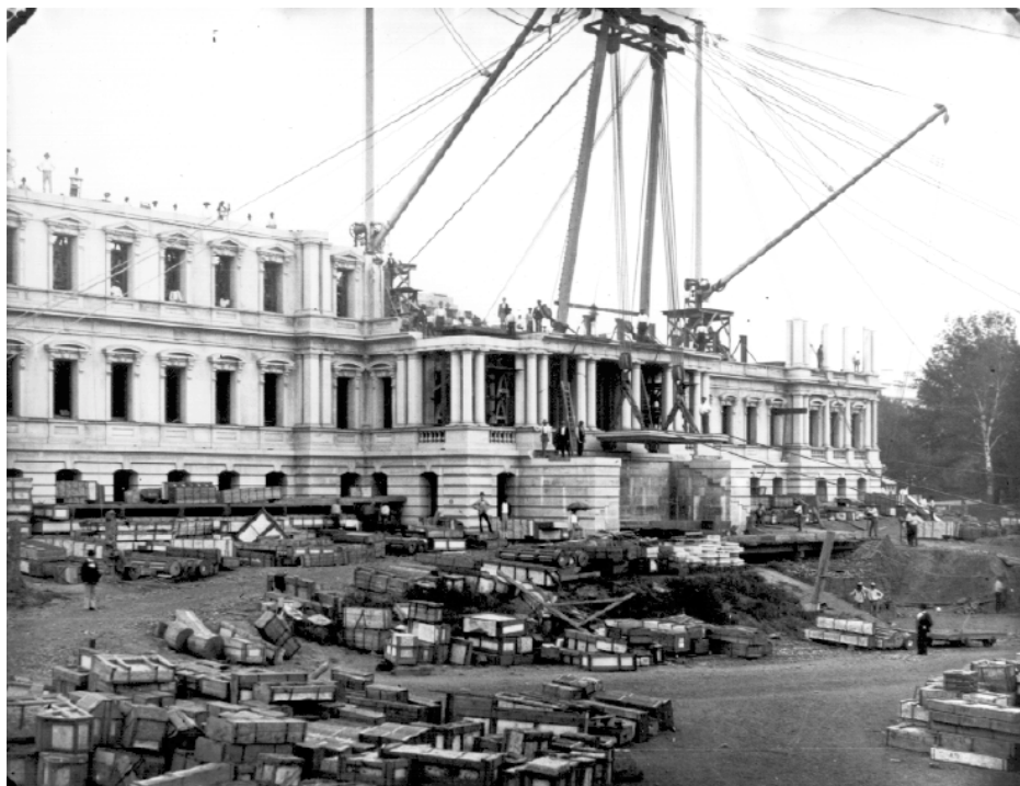
Fig. 3 Navy War Building under construction throughout the 1880s (National Archive, Washington, DC)
