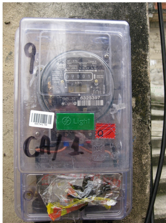
Figure 12 An electric meter disconnected as soon as it was installed became a subtle yet publicly visible protest of formal service provision in Saqualé.
