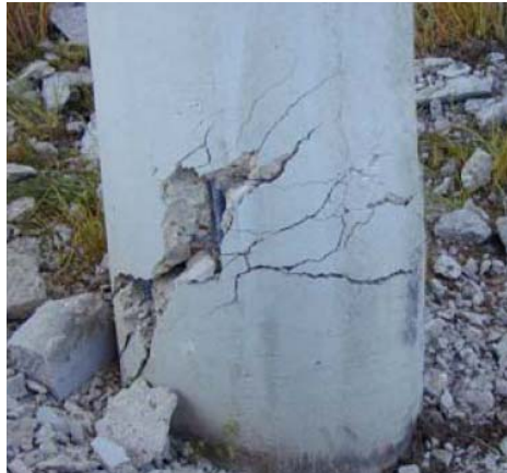
Figure 4.14 Spalling of Concrete Pier in the Collision Accident of Tyler, Texas (2004).
