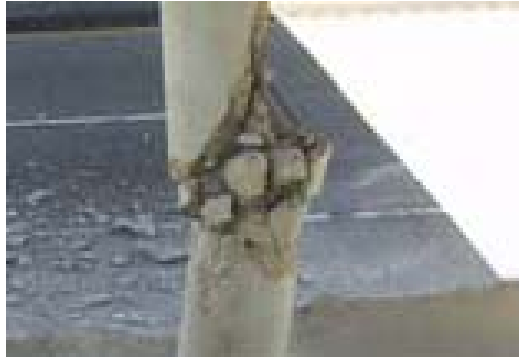
Figure 4.18 Severance of Rebars in the Pier Steel Cage in the Collision Accident of Tyler, Texas (2004).
