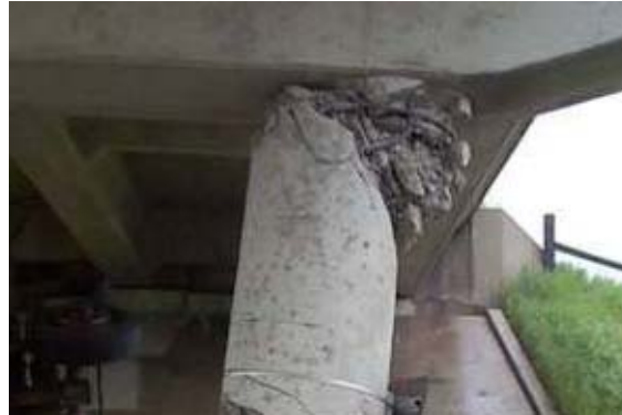
Figure 4.20 Plastic Hinge Formation in the Pier of 2003 Minnesota Collision Accident
