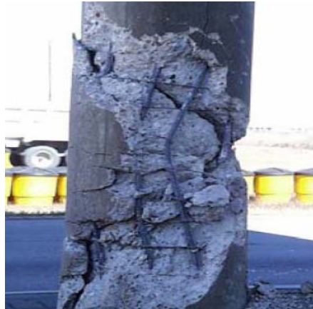
Figure 4.16 Breakage of Bridge Pier in the Collision Accident of Sealy, Texas (2004).
