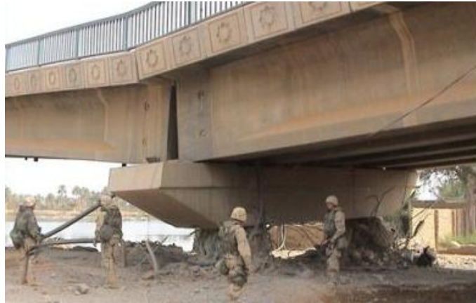
Figure 1.1 Bridge damaged by a relatively small amount of explosives during a terrorist attack.
