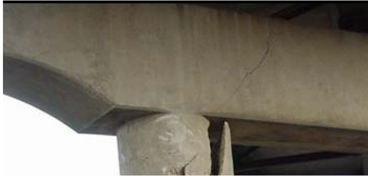
Figure 4.22 Damage of the Bent in the Collision Accident of Red Oak, Texas (2005)
