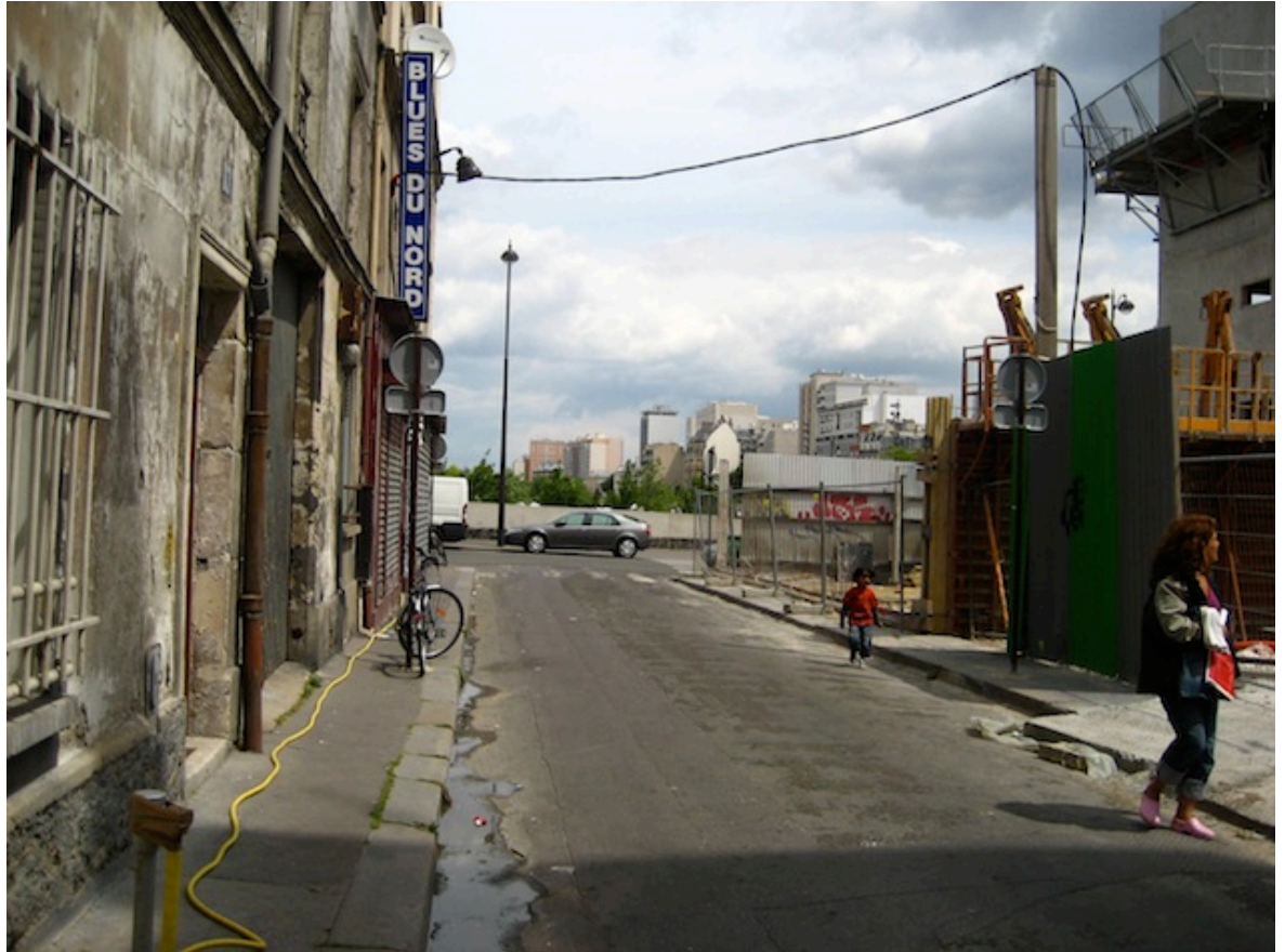
Figure 19: Street adjacent to the Jardins d'Éole, undergoing demolition. The apartment building and hotel on the left is slated for demolition (note the water-pump in the foreground, which is used by inhabitants whose apartments lack running water). On the right, new housing is under construction.
