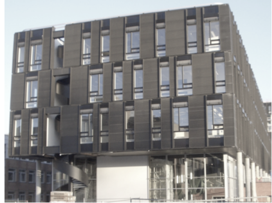
Figure 5. Building 4. New building of the Informatics Department at UiO, still under construction.
