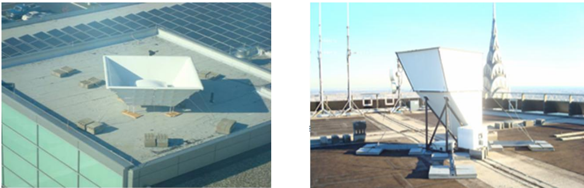
Figure 1-1, A radar wind profiler (left) mounted on the Liberty Science Center and a sodar wind profiler (right) mounted on a NYC high rise [1]
