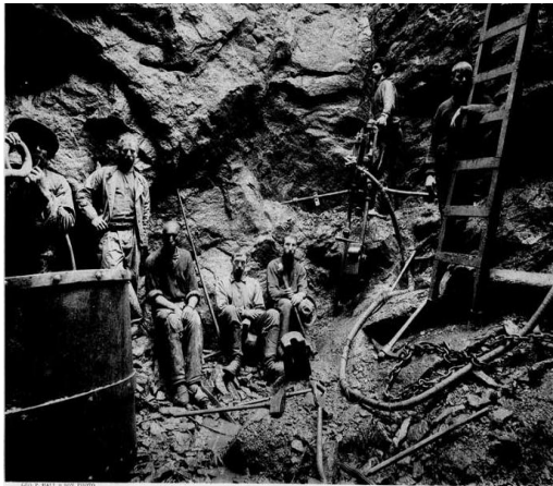
Figure 2.17: Excavating Shaft # 26, Photograph from City of New York Aqueduct Commissioner: Report on the New Croton Aqueduct, Reservoirs, and Dams: 1895-1907 , New York City Department of Environmental Protection Archive. Courtesy of DEP Archive.
