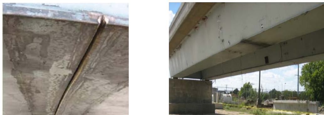
Figure 5.10 - Fracture view in the bottom flange
