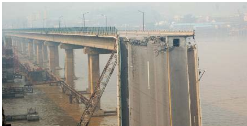
Figure 1.2 Collapse of Jiujiang bridge in June 2007 in China
